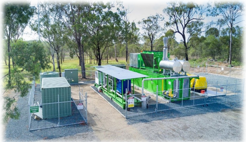
Benaraby, Gladstone Biogas to Power Project - Since 2016
